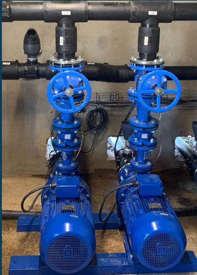
Pompes Lowara NSCE 40-250 – 15 kW
