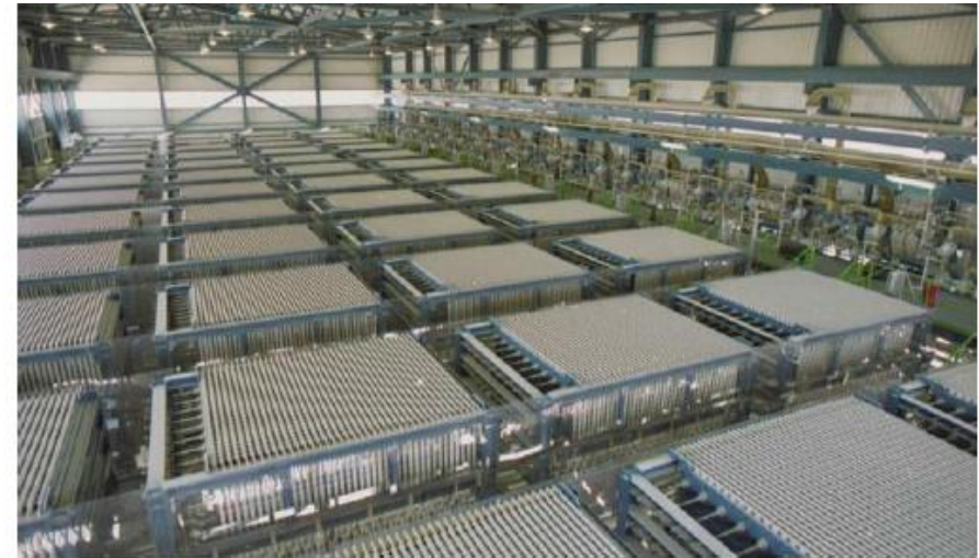
Chlor-alkali cell room – Uhde GmbH
